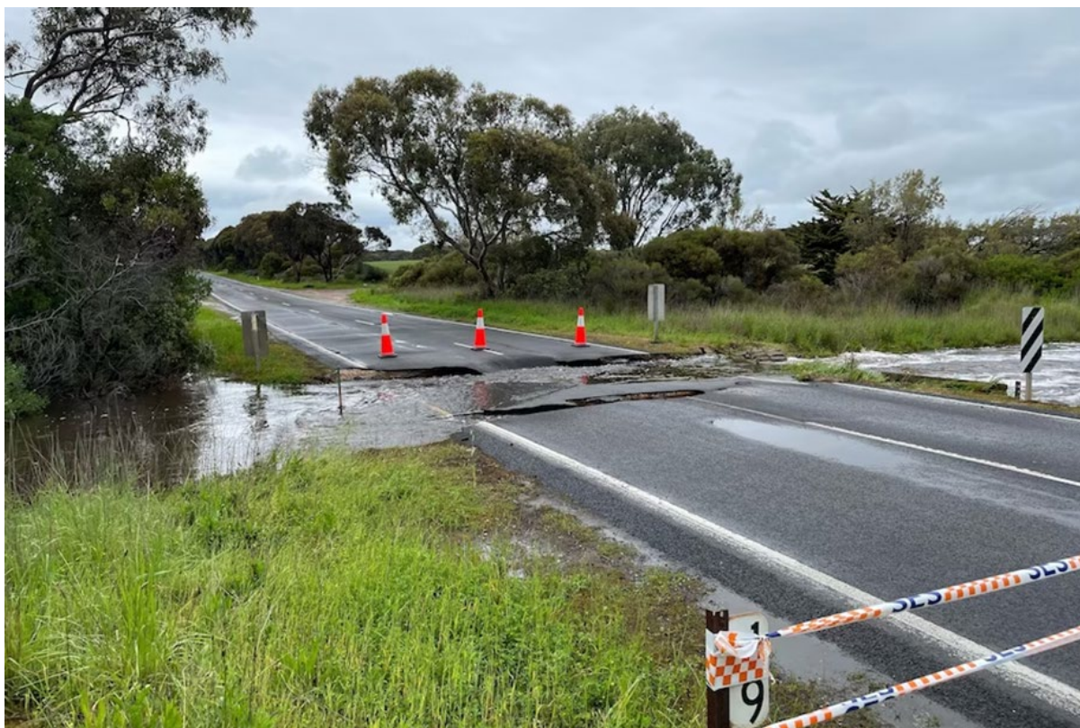
Figure 12 - Flash flooding damage to Hog Bay Road (Source: ABC News, 2022)
